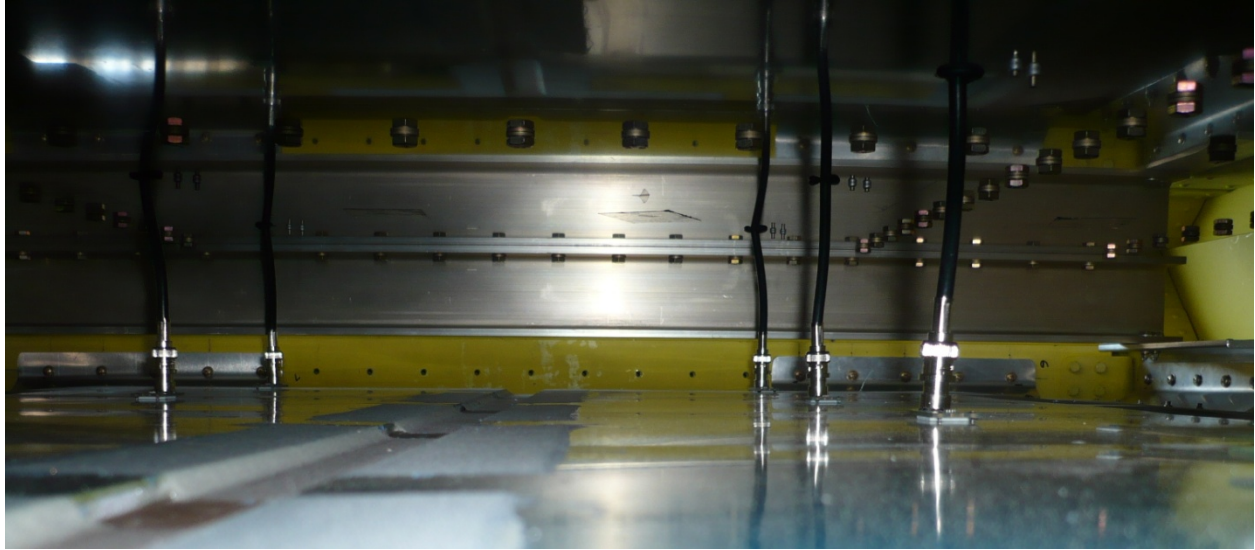
Figure 112. Photograph of the elliptical dipole array installed, cables passing through ground plane and connected to elements.
