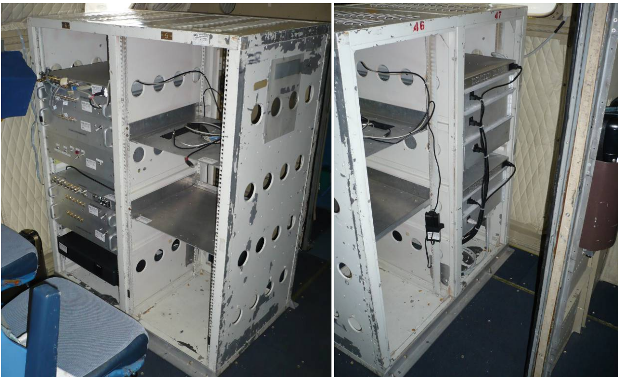
Figure 71. Front (left) and back (right) of accumulation radar rack on P-3.
