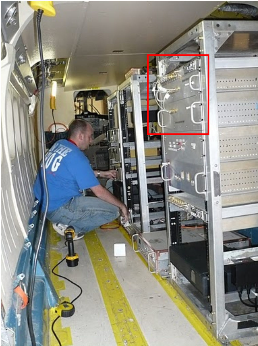
Figure 63. Photograph of the installed accumulation radar (highlighted).
