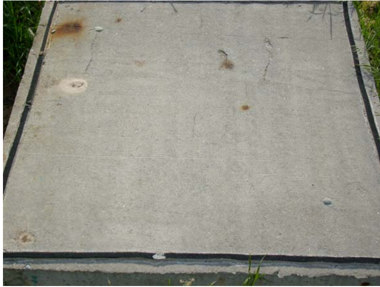
Figure 3.90 – Field test specimen Conv. (1) at week 205, showing cracking, spalling, and heavy staining on portions of the surface.
