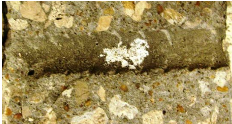
Figure 3.140 – Initiation Beam Test. Specimen with zinc-coated reinforcement after autopsy (B-Zn-45N-10) showing visible interior staining of the concrete.
