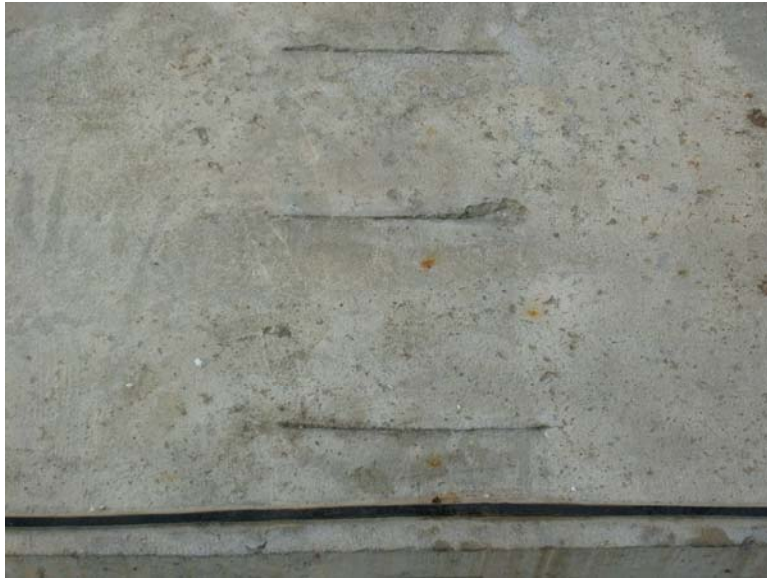
Figure 3.91 – Field test specimen ECR(DCI) (1) with simulated cracks at week 179, showing light staining on the surface.
