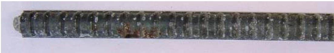
Figure 3.139 – Typical corrosion at initiation on conventional steel.
