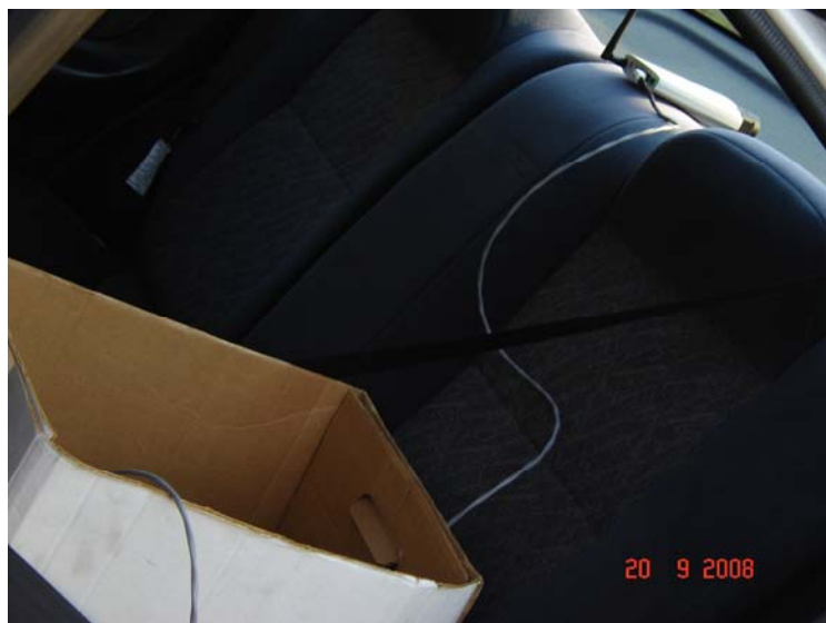
Figure 5.10: Power Cable for the IP Camera
