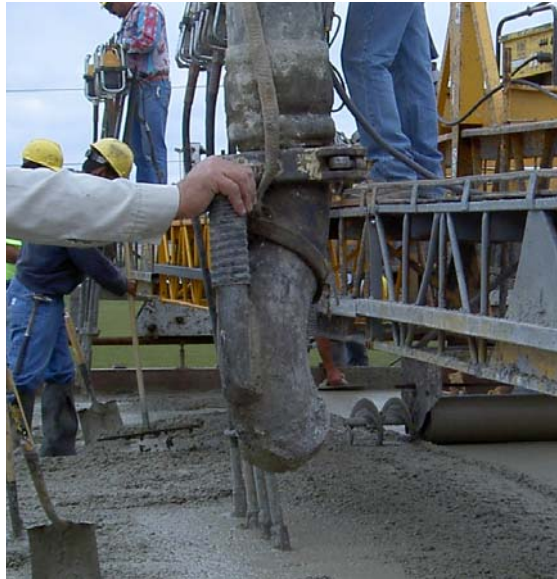
Fig. 5.12 – Elbow fitted to the end of the pump hose to limit air lose through the pump.
