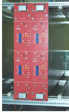
Figure 2.14: Two CAEN Power Supply Modules (PSM, CAEN A4601H model) in a crate.
