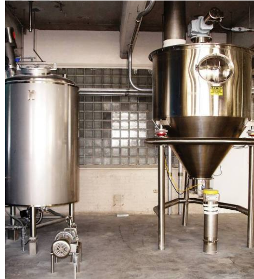
Exhibit 11: 400 Gallon Tank and K-Tron Feeder
