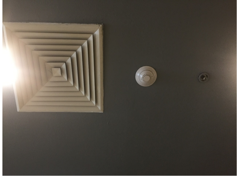
Diffuser, sprinkler and smoke alarm not following NFPA distance specifications
