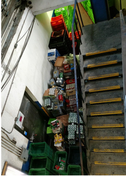
Fire Hazard - Objects covering exit
