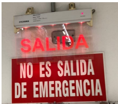
Figure 8. Contradictory Exit signs (By Authors)
