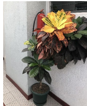
Figure 3. Fire extinguisher covered by plant, inhibiting accessibility
