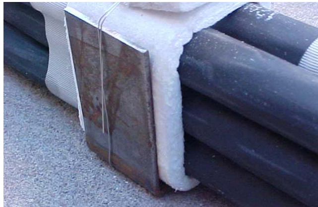
Figure 3-7 Multiple Cable Bundle, Side View
