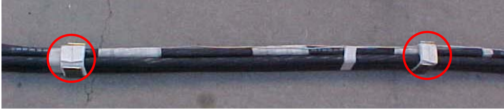
Figure 3-9 Multiple Cable Bundle, Overhead View
