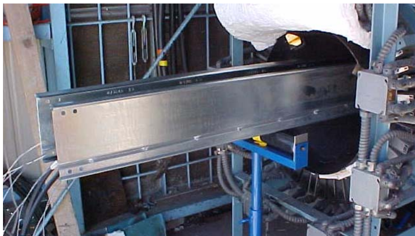
Figure 3-3 Single Cable Experiment in PENLIGHT, side view
