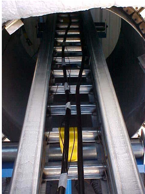
Figure 3-2 Single Cable Experiment in PENLIGHT, front view
