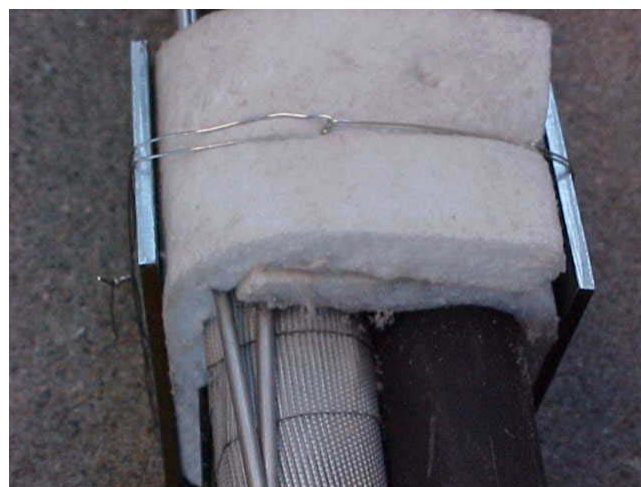
Figure 3-8 Multiple Cable Bundle, Top View
