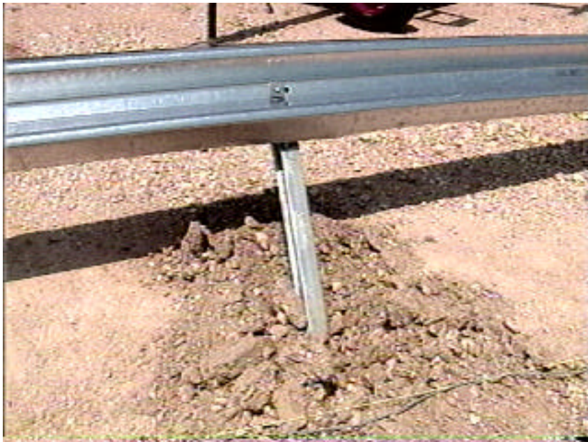
Figure 105: Post-test close-up on post.
