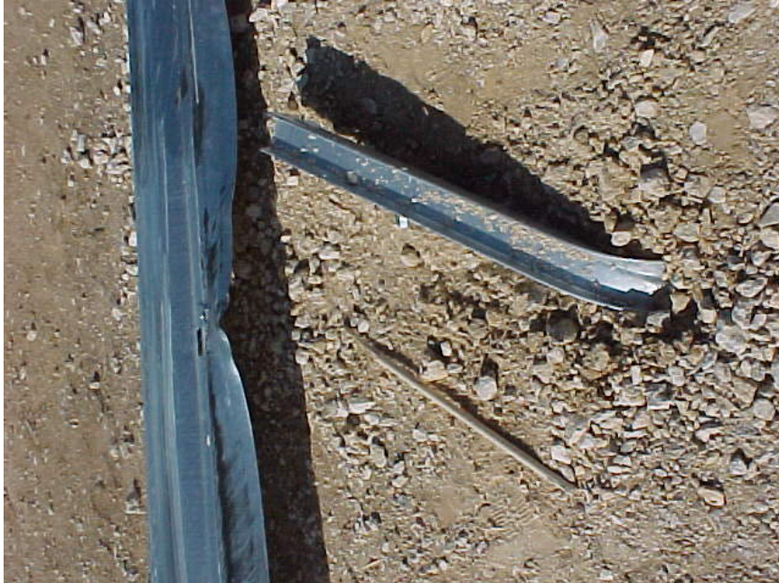
Figure 56: Guardrail tear initiated at a post.(9)
