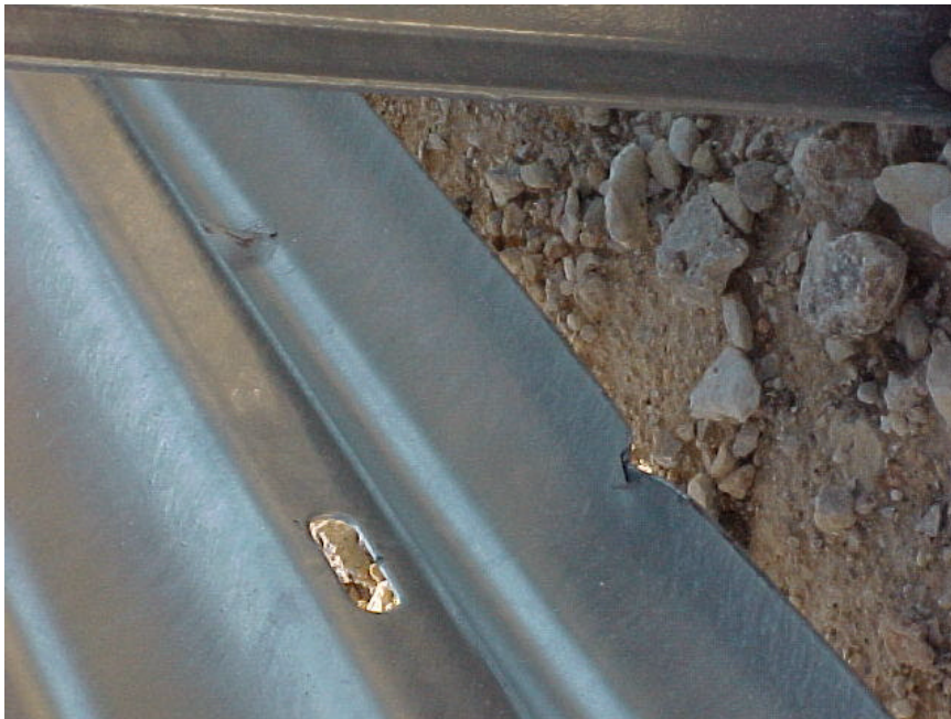
Figure 57: Rail deformation at a post.(9)
