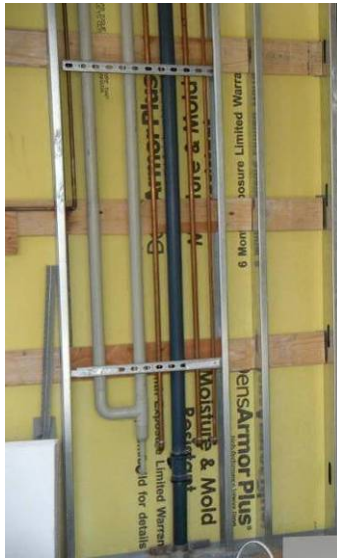
Figure 24: Prefabricated Laboratory Tempered Water, Hot water, Cold Water, Lab waste Lines
