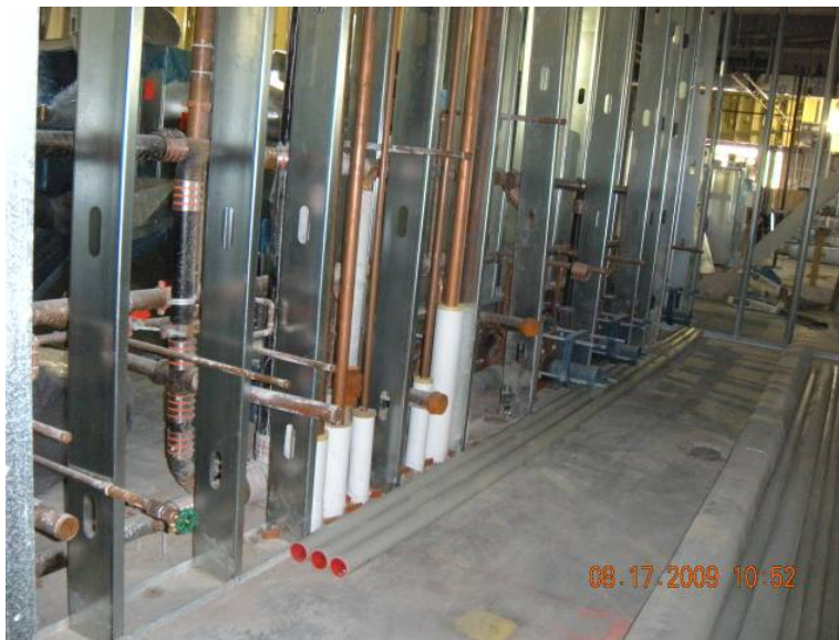
Figure 25: Prefabricated horizontal runs at the bathroom
