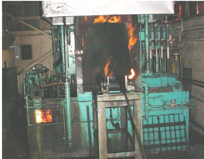
Fig. 19 Gas fired Furnace
