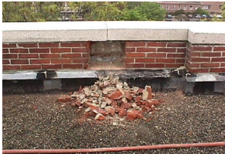
Figure 7.4. Pre-cast concrete parapets and bricks to be removed and replaced
