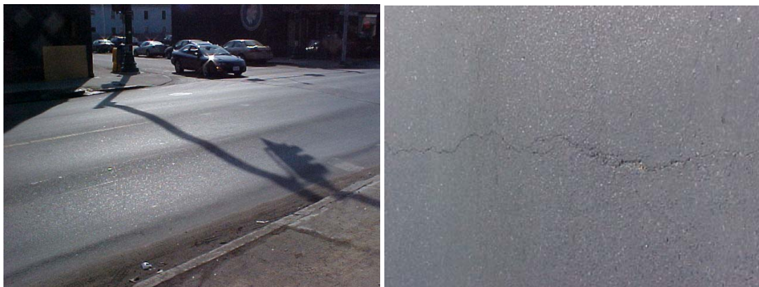
Figure 22: Examples of Problems in Pavement Quality
