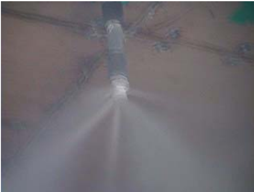
Photograph 6. CO2 Discharge into Enclosure
