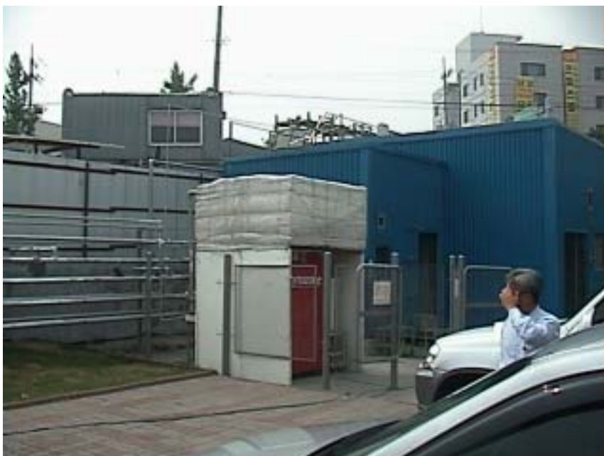
Photograph 2. Low Pressure CO2 Storage Container
