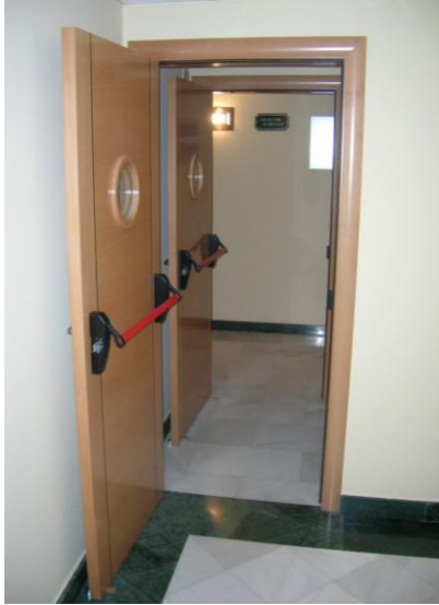
Fig. 4-11. Blocked opened doors in a vestibule separating hotel room corridor from a stairwell in a hotel
