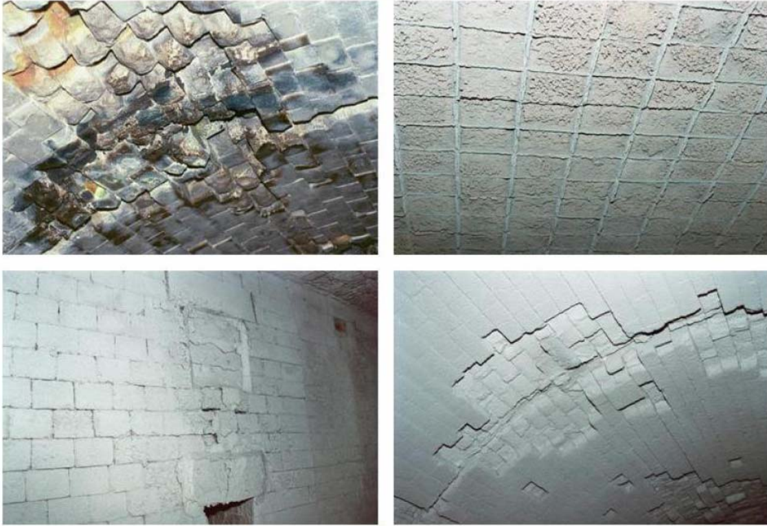
Figure 5.25 - Spalled and corroded furnace refractory walls [12]
