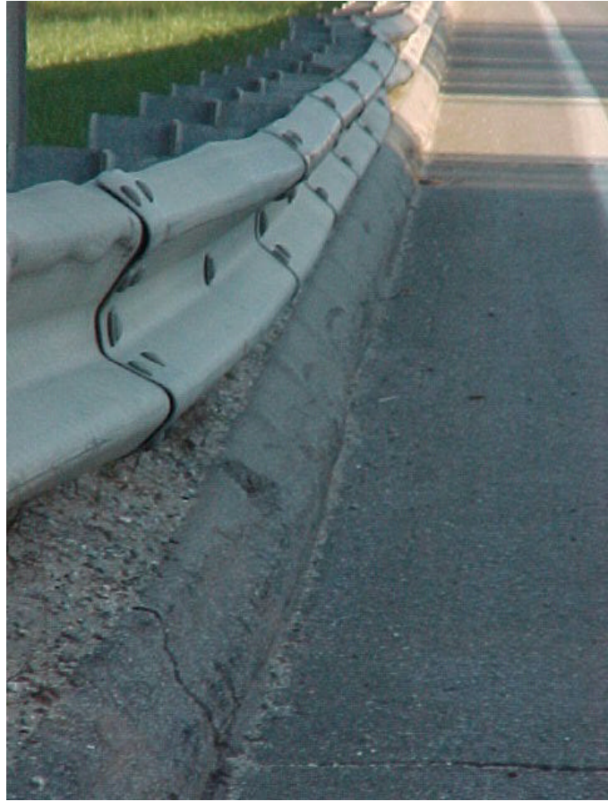
Figure 1.2: Sloping curb installed flush with a strong-post w-beam guardrail on a 90 km/hr two-lane rural roadway in Maine.
