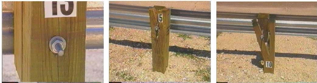
Figure 2.12: Posts split vertically during TTI test 404201-1 along pre-existing splits in posts. (32)
