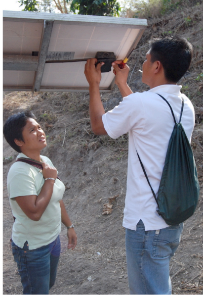
Figure 1 - Solar Home System PV Component and BGET Technicians
