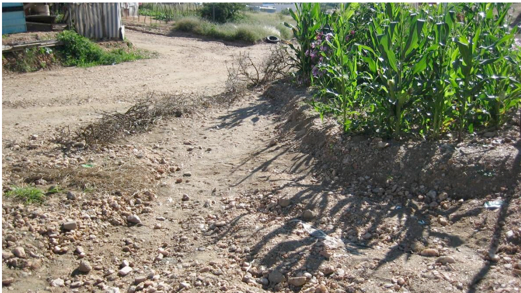
Figure 10: Erosion Damage at Site #3 Before Construction
