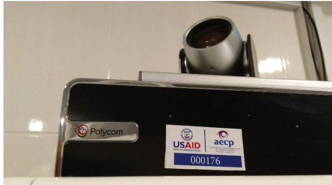
Figure 17: Polycom RealPresence Group 700 system box and camera
