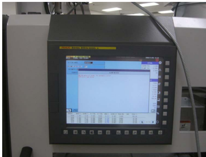
Figure 23: Molding Machine Central Control
