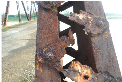
Figure 1: Corrosion on infrastructure. 3
