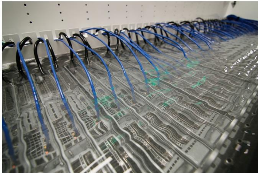
Figure 11: Liquid Submerged Servers
