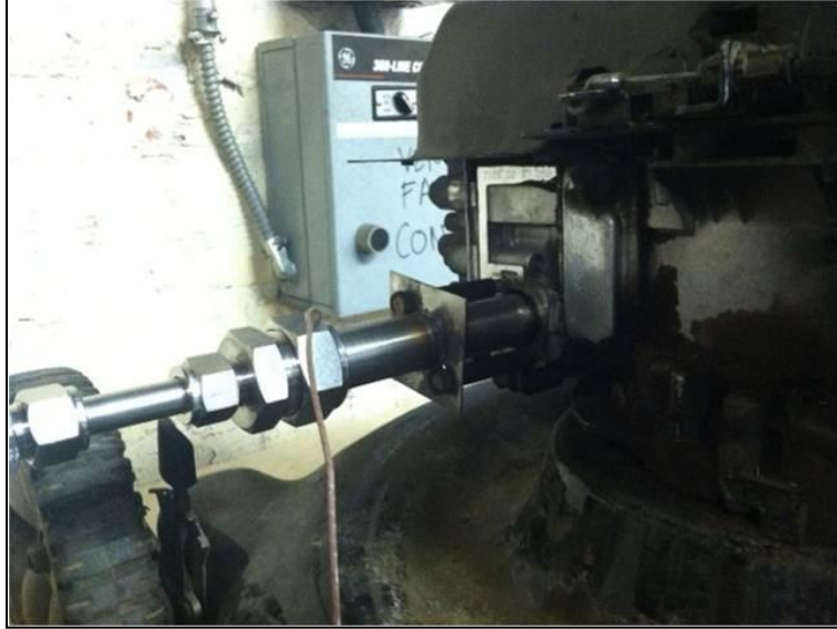
Figure 48: Exhaust outlet connecting to cooler
