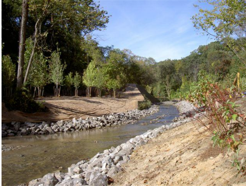
Figure 8 - Stream bank showing the use of riprap for erosion control (Michigan Department of Water Resources, 2011)
