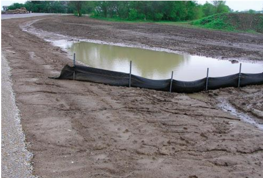
Figure 6 - A properly installed silt fence retaining run-off for sedimentation and filtration to occur (Carpenter, 2006)
