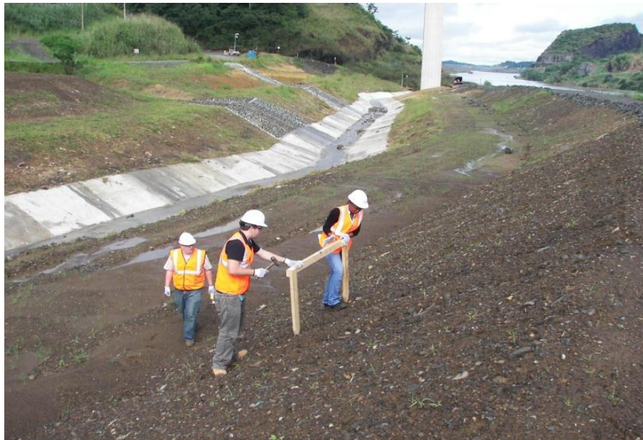
Figure 15 - Site 1 with steep slope and no BMP at the time of erosion bridge installation (Photo Credit: Tomás Antonio Edghill, 2011)
