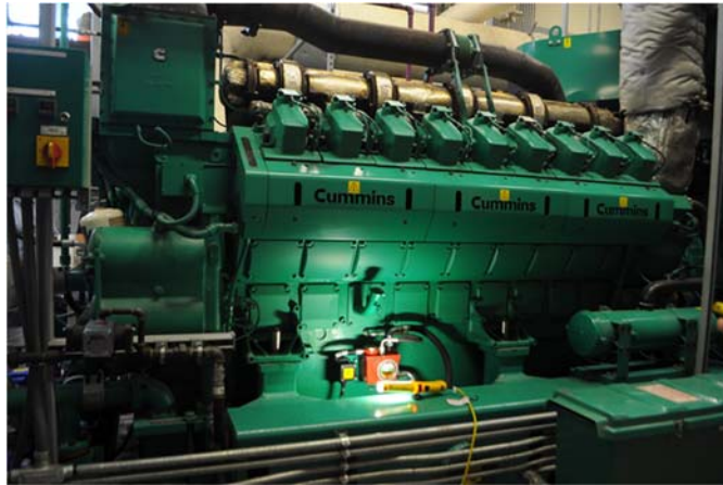
Figure 19 - Clark Universities 2MW Diesel Engine
