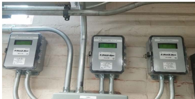
Figure 22 - E-mon Demon Smart Meters WPI Powerhouse
