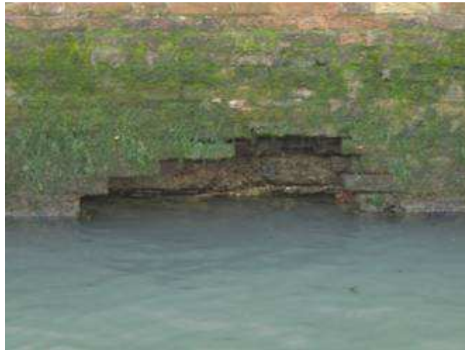
Figure 6: Canal Wall Damage
