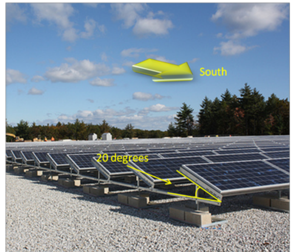
2.5 Megawatt array in Westford, MA developed by Nexamp
