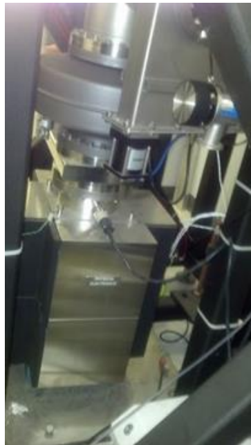
Figure 28: Physical Electronics 640 I/s Ion Pump
