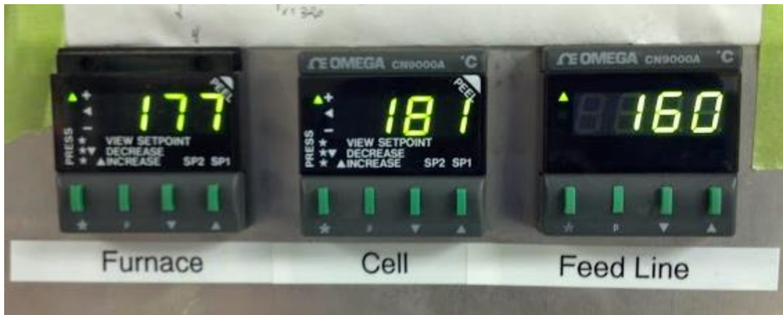
FIGURE 44: TEMPERATURE CONTROL BOXES
