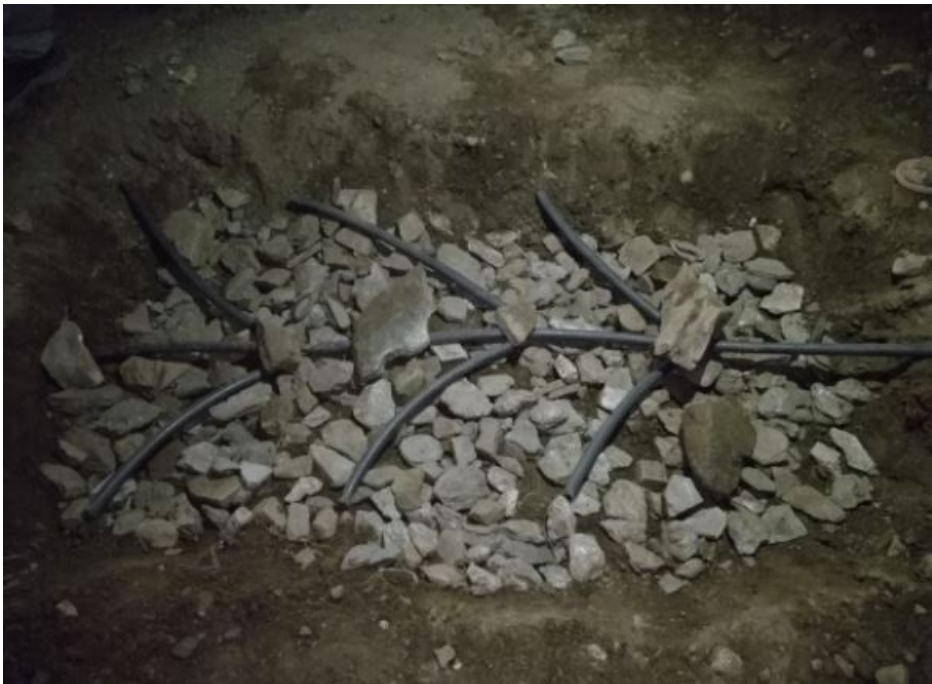
Underground heating system in the nursery prototype
