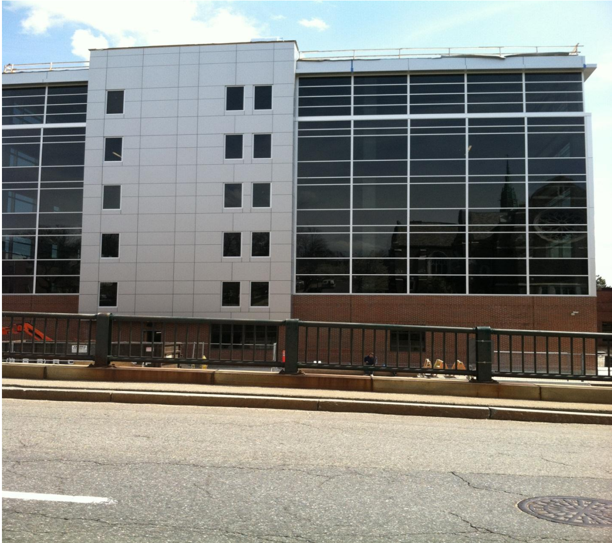
Figure 1: Street view of the west elevation of the MCPHS building during construction.
