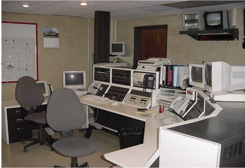
Figure 9: Motorola Centracom II Communication Consoles (Motorolla) [55]
