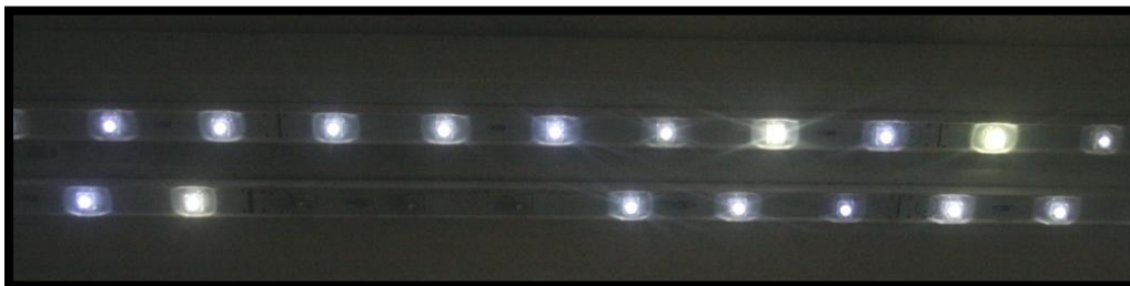
Figure 1: LED Light Fixture in Stairway
