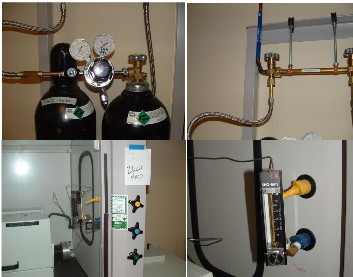
Figure 43 - Nitrogen Supply Valves
