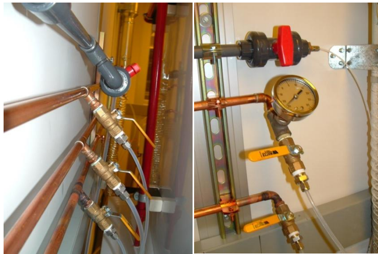
Figure 31 - Hood Supply Lines (Left) and Spin Coater Supply Lines (Right)
