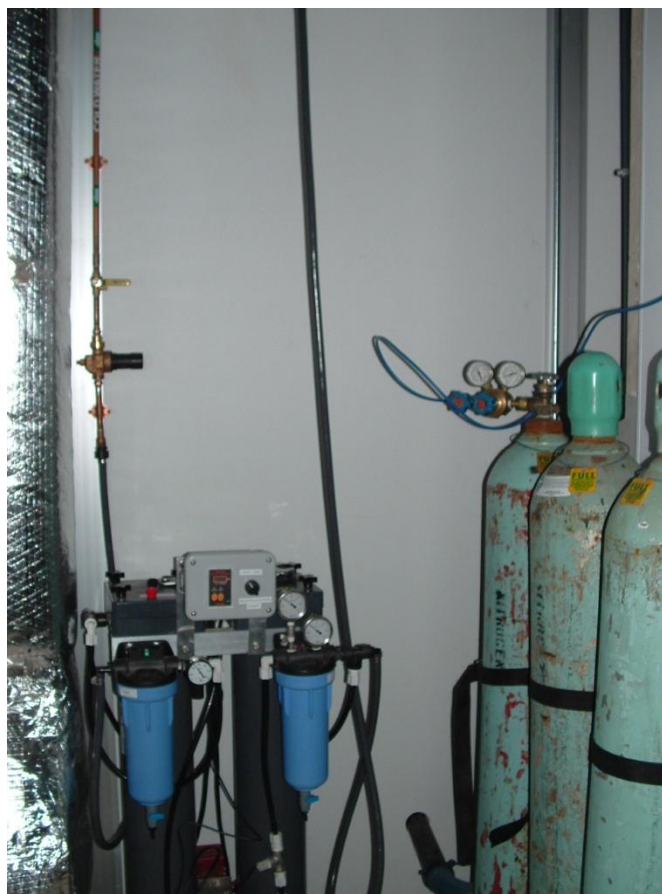
Figure 28 - Clean Room Supply Inlet
