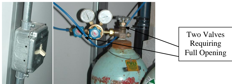
Figure 30 - Vacuum Switch and Nitrogen Gas Valves
