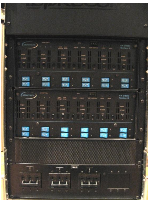
Figure 1 - Front of a typical dimmer rack.
