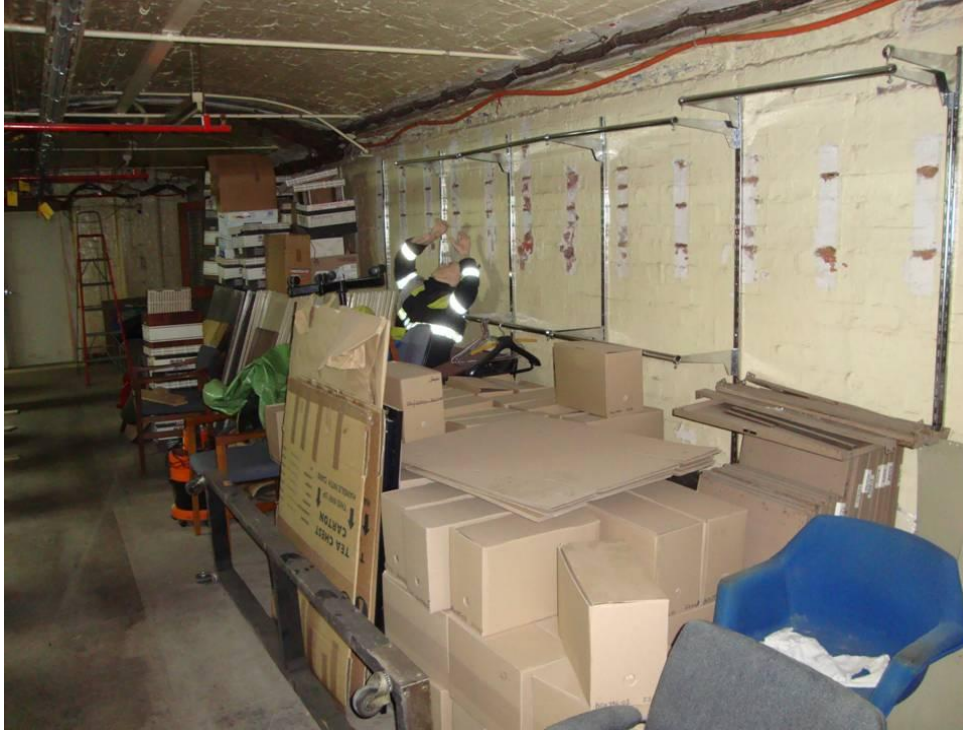
Figure 6.5 – An Example of Poor Perimeter Storage
