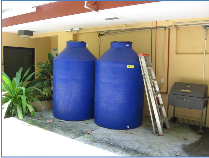
Figure C-3: Photo of 550 Gallon Tanks for Storage of Potable Water on BCI, Jan. 13, 2010
