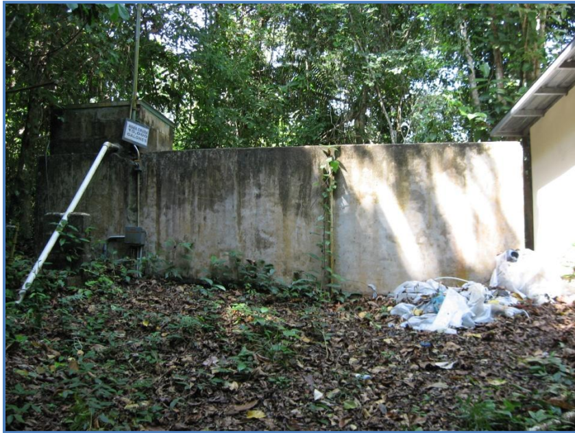
Figure A-6: 15,000 Gallon Concrete Tank
