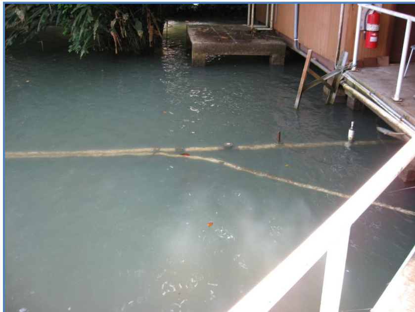
Figure A-2: Pipeline Leading from Intake to Pumps
