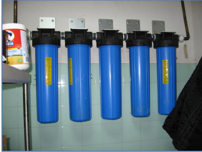
Figure B-3: Filter in Kitchen
