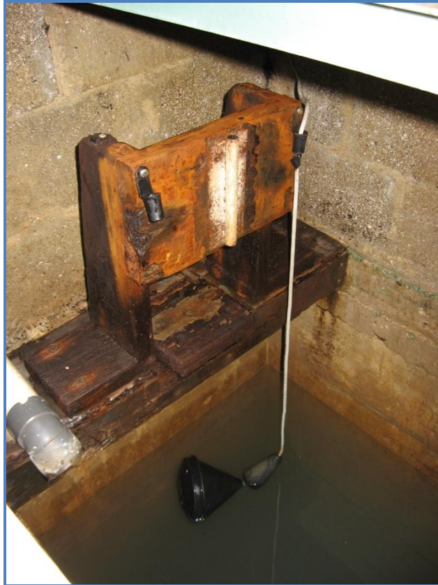
Figure A-7: Buoy Water-level Sensor in Concrete Tank
