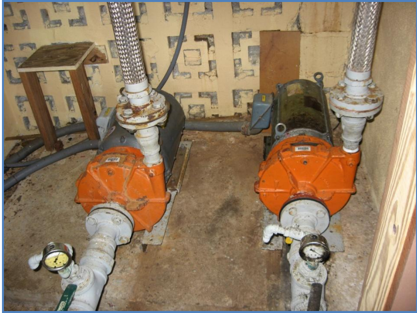
Figure A-3: Water Pumps at Docks
