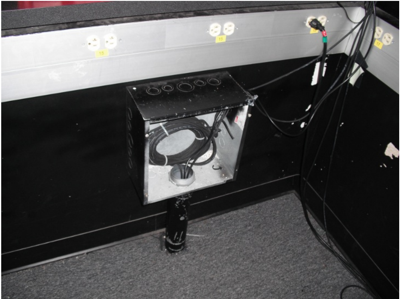
The box inside the booth through which cables are run into the green room
