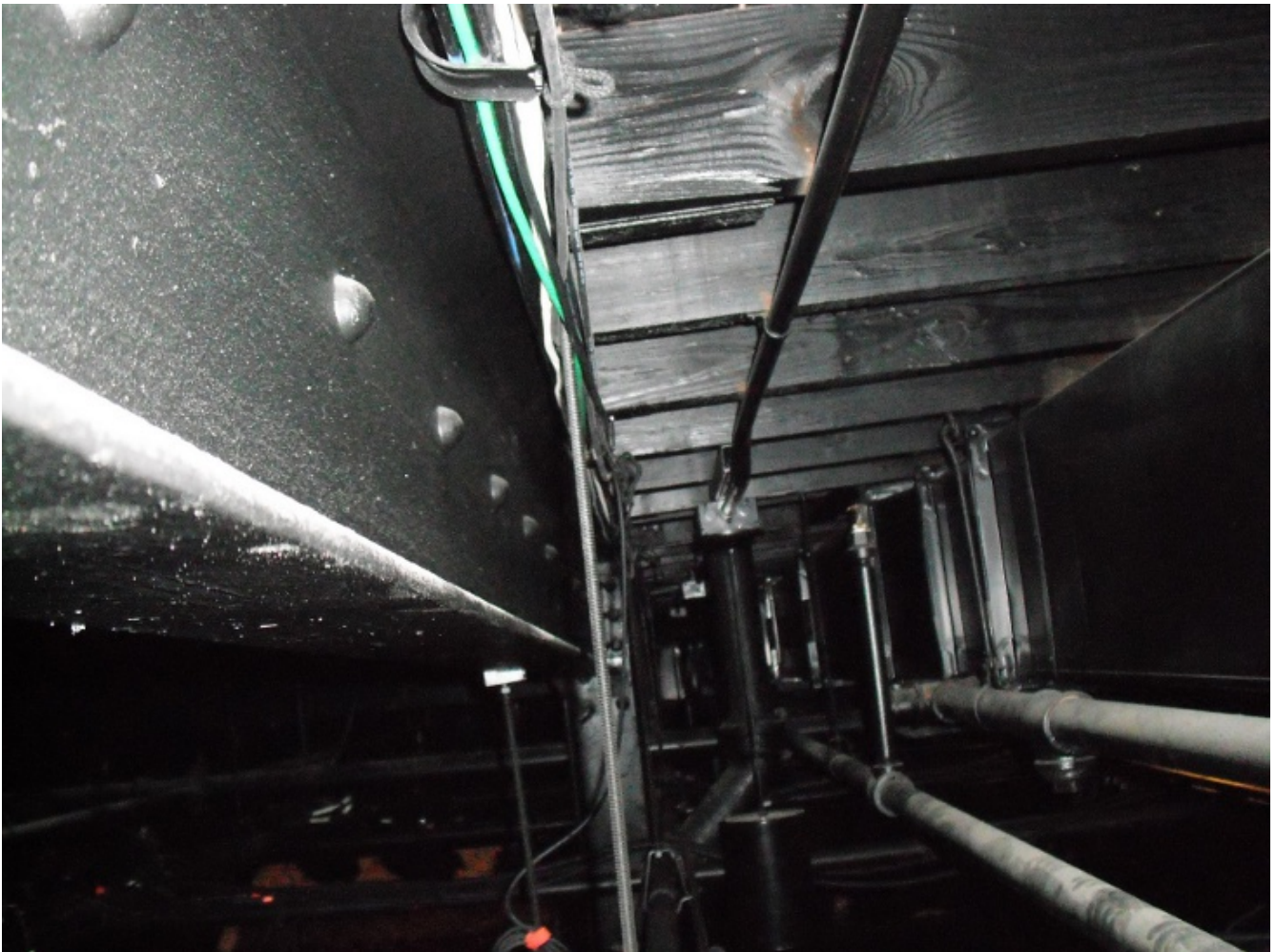
The trough through which permanent cables are run
