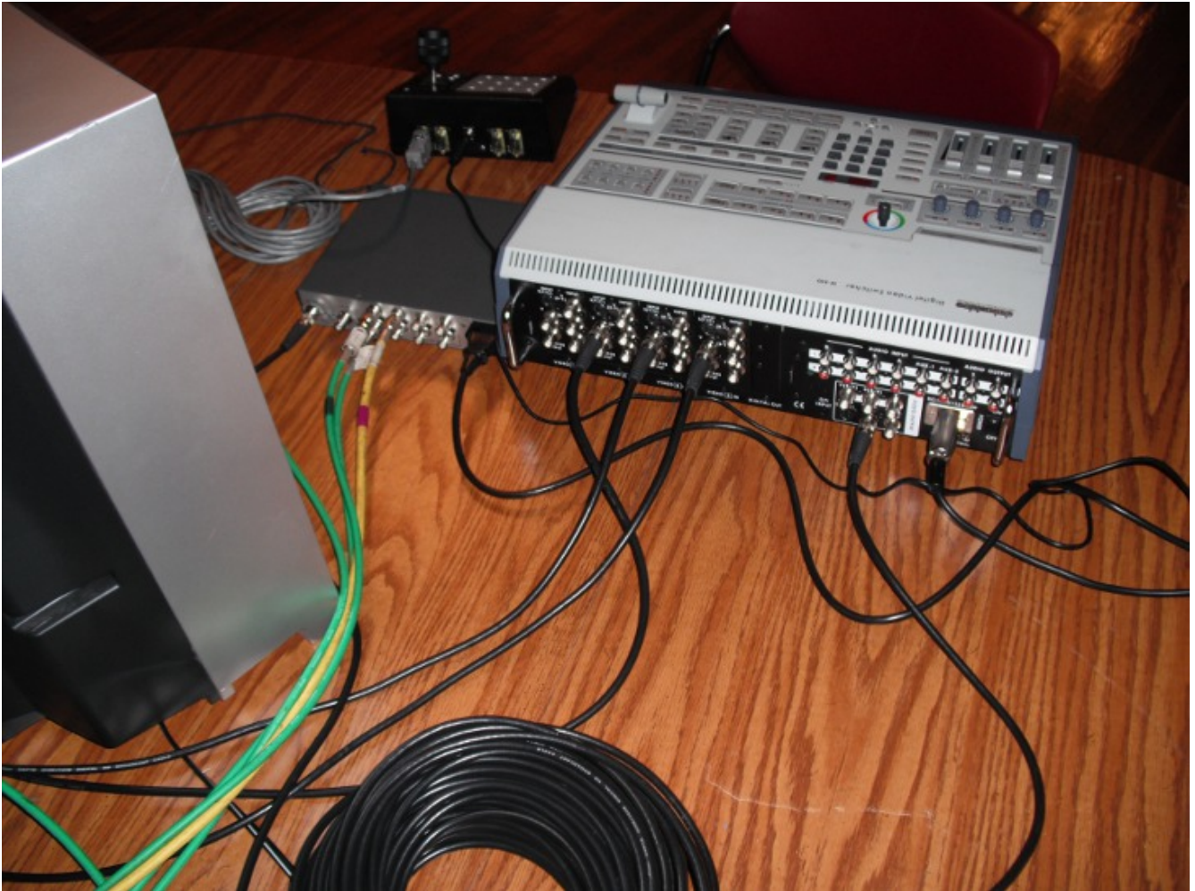
The back side of the control setup
