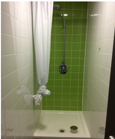
Figure 21: Croydon Council shower
