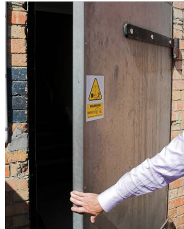
Fig. 4.5.4F – Warning Signage on Rear Door
