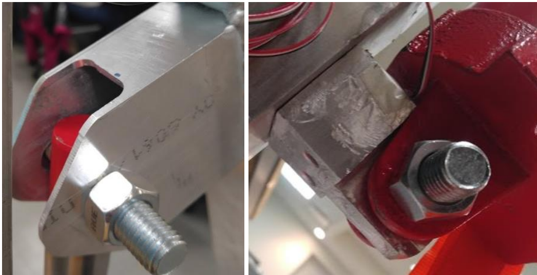
Figure 60: Hydraulic Pump Supports
