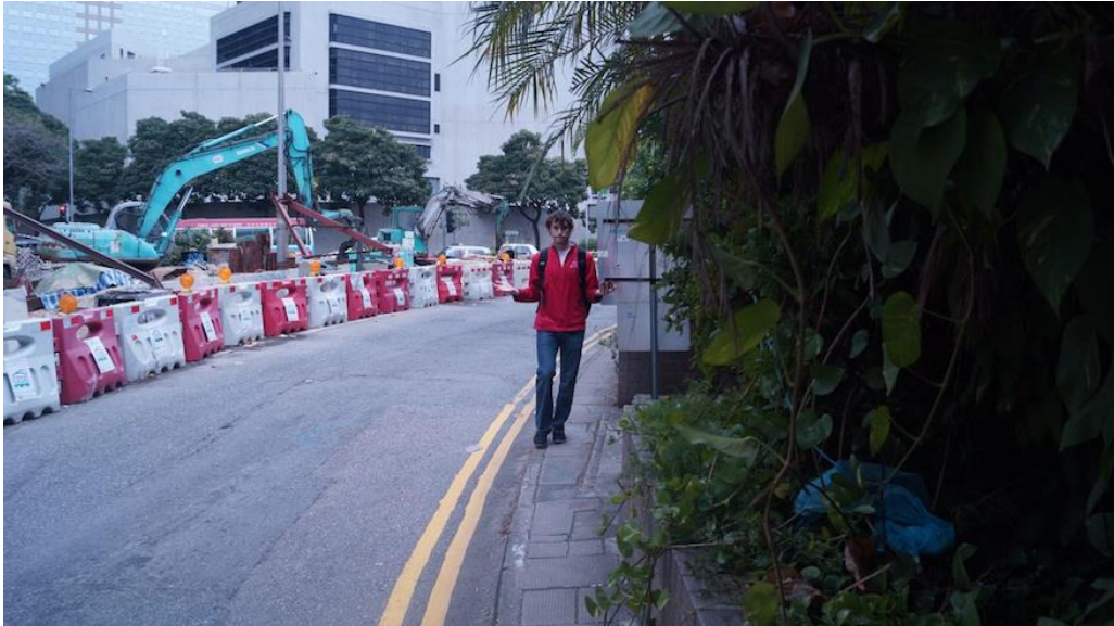
FIGURE 44: UNSAFE SIDEWALK AVAILABLE TO PEDESTRIANS. (COURTESY OF ALFRED SCOTT)
