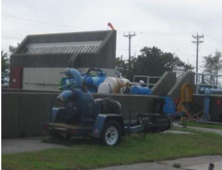
Figure 6. 1: Portable Pump Motor
