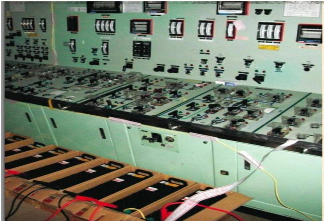
Figure 3. Temporary batteries were used to read crucial instruments throughout the station blackout (Strickland, 2011).
