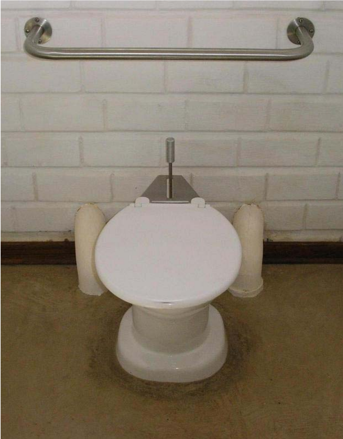
Figure 4.4: Interior installation of Enviro Loo dry toilet system at the HRDC.
