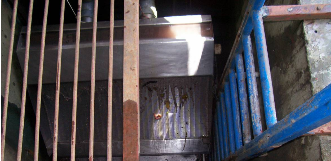
Figure 30: Final Filter Before Wastewater Enters Treatment Pond
