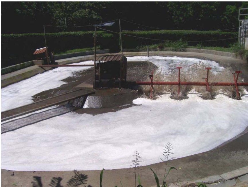
Figure 31: On-Site Wastewater Treatment Facility
