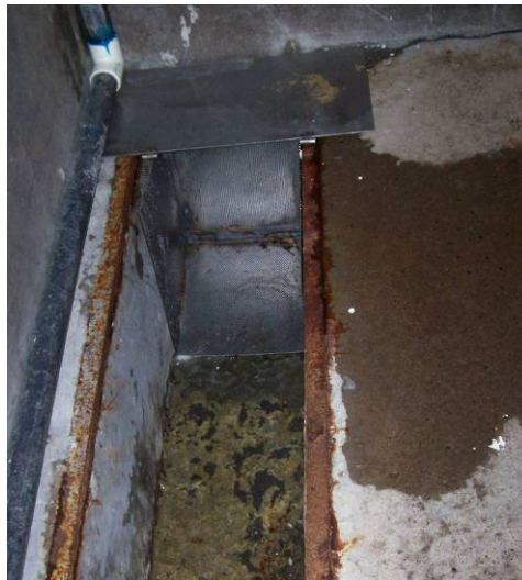
Figure 29: Typical Filter at Exportadora PMT
