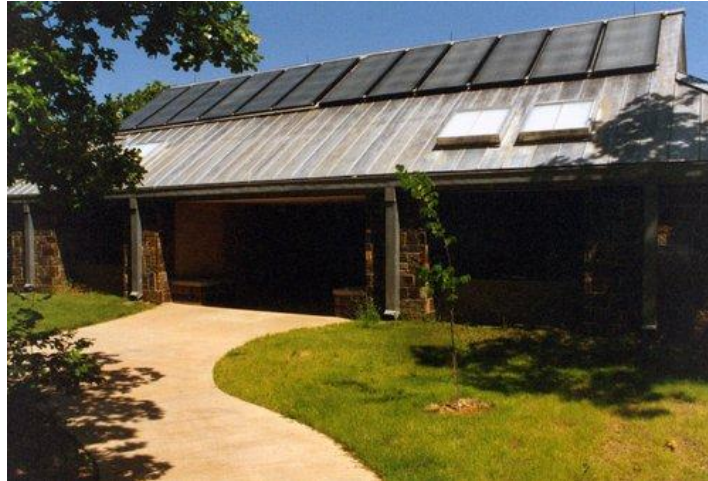
Figure 2.9: Large Comfort Station Solar Hot Water System at Buckhorn Campground (National Renewable Energy Laboratory, 1998)
