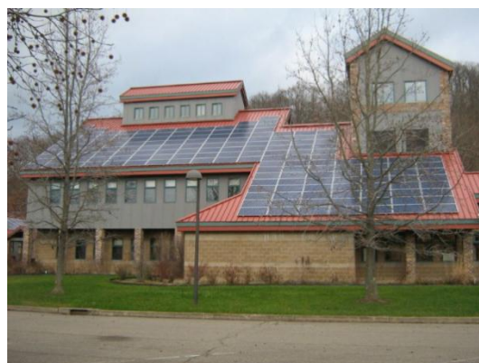
Figure 2.6: 59 kW Photovoltaic System at Wayne National Forest Headquarters (Sound, 2010)
