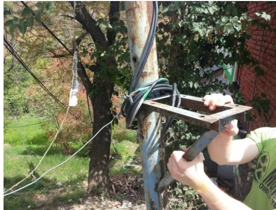
Figure 1. A broken solar street light with a missing battery
