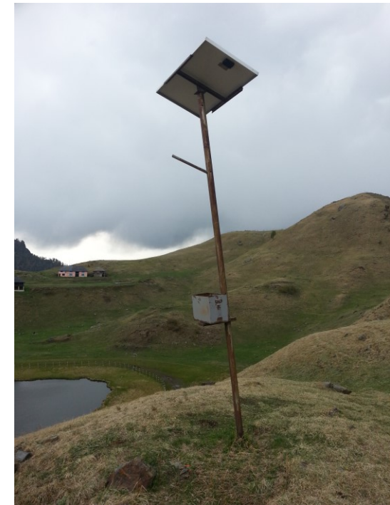
Figure 8. Broken light at Prashar Lake
