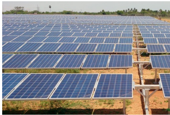
Figure 3. A 4 MW PV installation in Tamil Nadu, India (Vinaykumar8687, 2014) (Wikimedia Commons)
