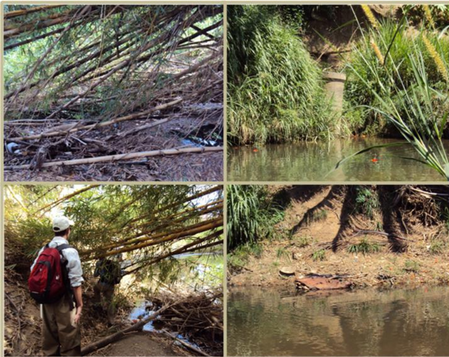
WPI-RP-1: (top and bottom left): Bamboo blockages; (top right): Drainage pipe; (bottom right): Metal pollutants
